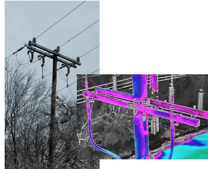
Left: Ice on trees in contact with power lines Right: Infra-red scanning of pole-top equipment using a drone
