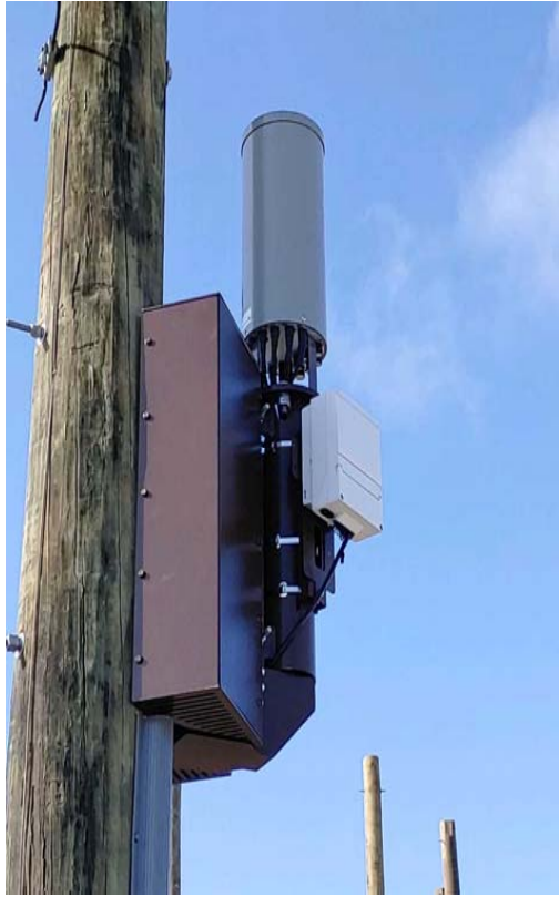
CPS Wood Pole "BEFORE"
