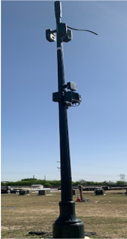
Valmont Decorative Streetlight BEFORE
