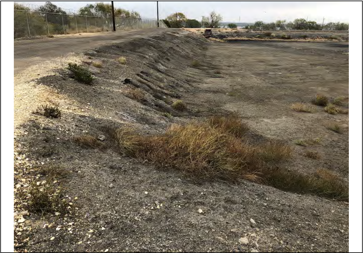
Photograph: 17 North Bottom Ash Pond – standing on northwest corner – facing east. Photo taken 12/15/2020.
