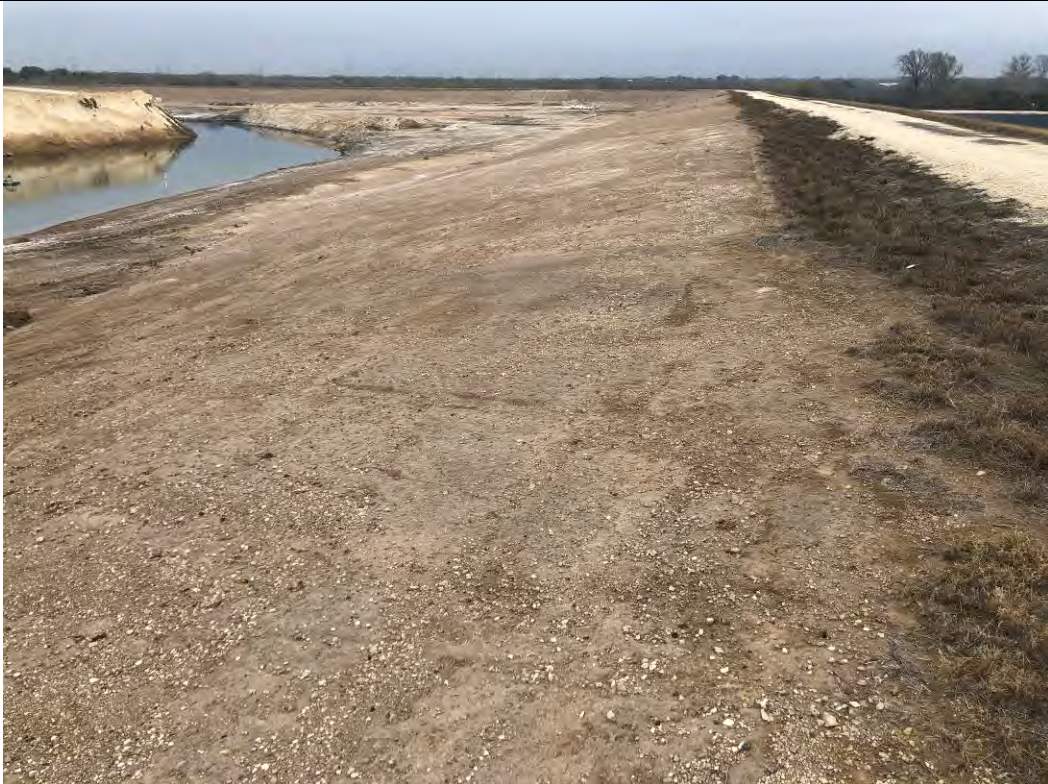
Photograph: 8 Fly Ash Landfill – standing on southeast corner – facing north. Photo taken 12/15/2020.
