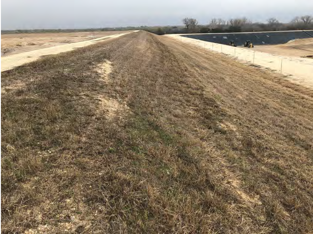
Photograph: 7 Fly Ash Landfill – standing on southeast corner – facing north. Photo taken 12/15/2020.
