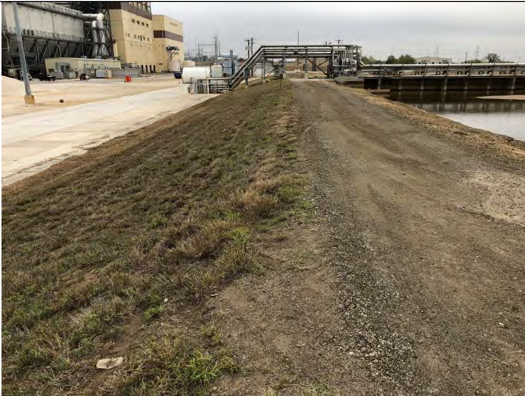
Photograph: 32 South SRH Pond – standing on the southwest corner – facing north. Photo taken 12/15/2020.
