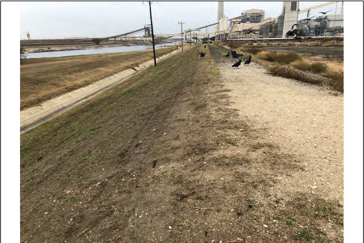
Photograph: 23 South Bottom Ash Pond – standing on southeast corner – facing west. Photo taken 12/15/2020.
