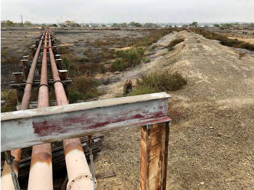
Photograph: 20 North Bottom Ash Pond – standing on southwest corner – facing east. Photo taken 12/15/2020.
