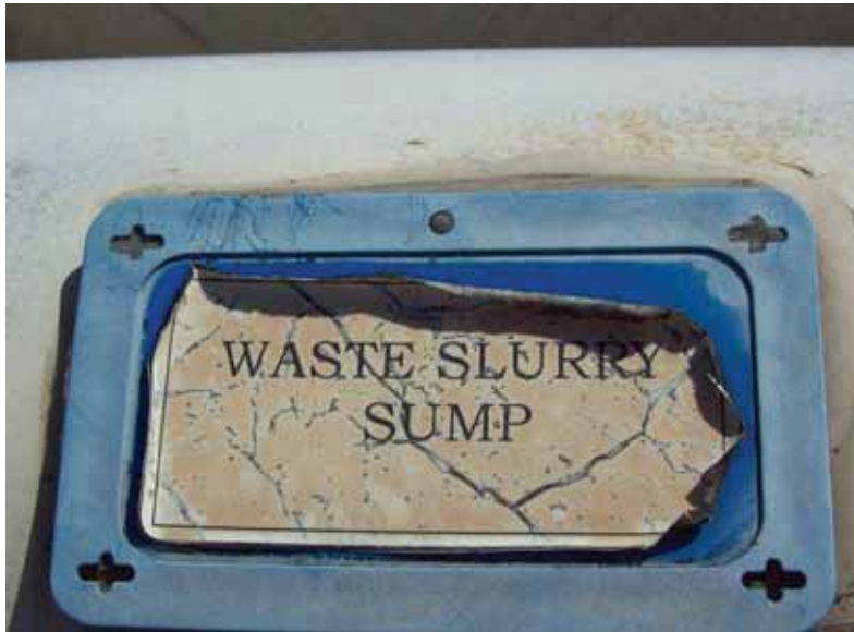
Photo 29: Label for inlet pipe in Photo 28.
