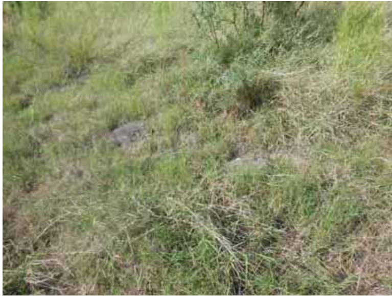
Photo 94: Loose soils on east embankment exterior slope.
