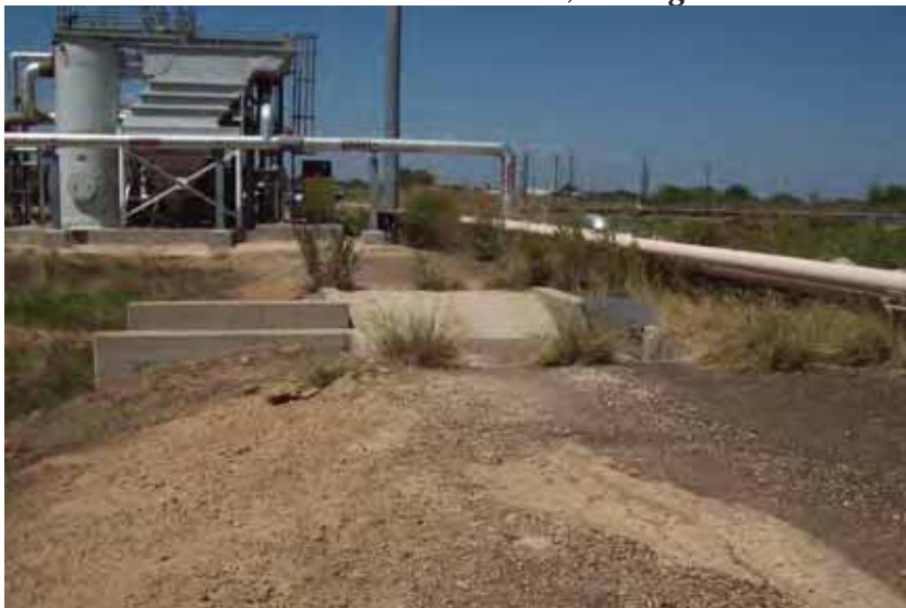
Photo 75: SP - Spillway between SRH Pond and South Bottom Ash Pond at west embankment crest, looking north.
