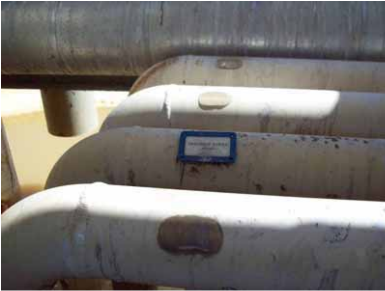
Photo 37: Labels for right four 4-inch-diameter inlets shown in Photo 34.
