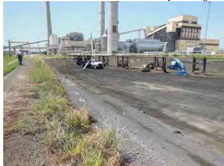
Photo 68: SP – South embankment exterior slope, looking west. Note equipment working in pond to replace inlet piping.
