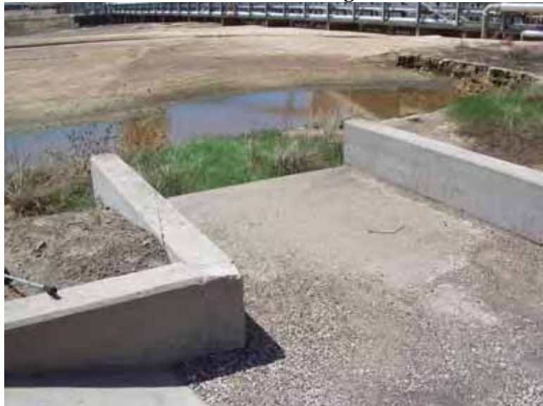
Photo 7: Spillway between SRH Pond and South Bottom Ash Pond at east embankment interior slope, looking west.
