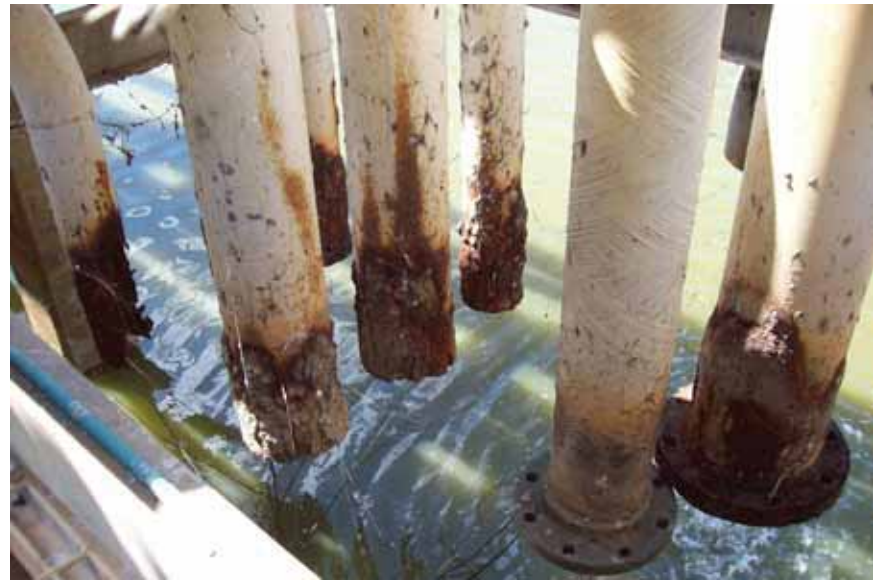
Photo 38: Nine outlet pipes into SRH-north, looking north.
