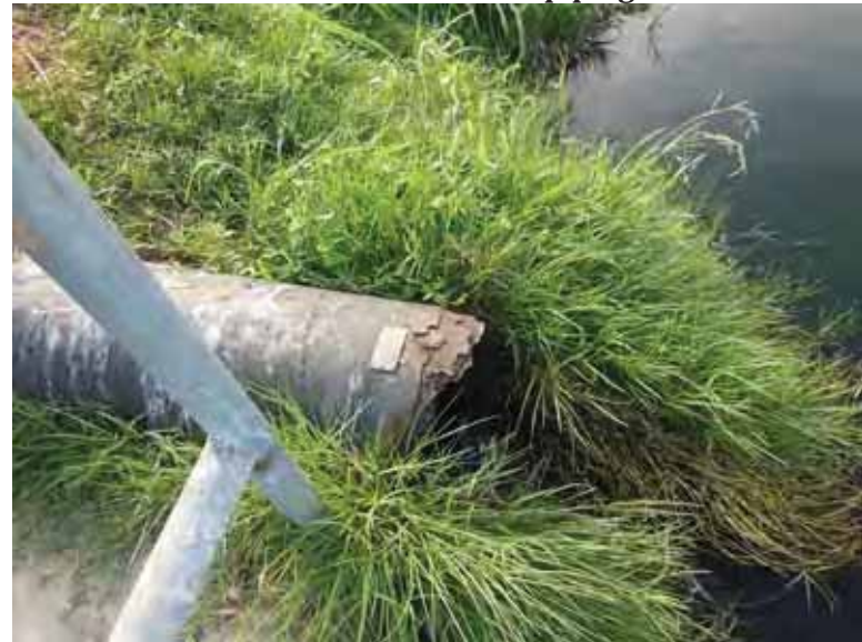
Photo 88: NP - 12-inch-diameter piping at outfall 103A.
