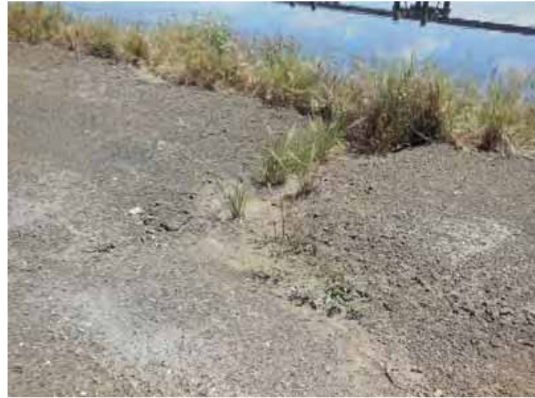
Photo 38: NP - Erosion rill in ash material at west embankment interior slope.
