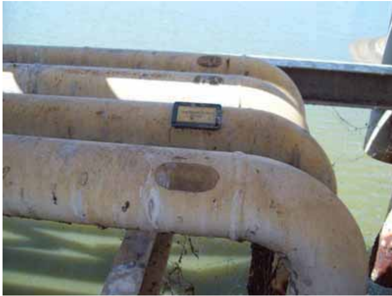
Photo 41: Labels for left four 4-inch-diameter inlets shown in Photo 38.
