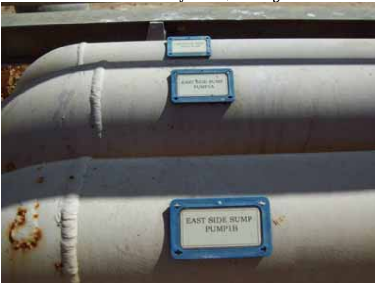
Photo 35: Labels for middle three 6-inch-diameter inlets shown in Photo 34.
