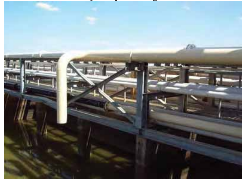
Photo 44: 8-inch-diameter metal SRH-north inlet pipe labeled "Plant Drain System III", looking southeast.
