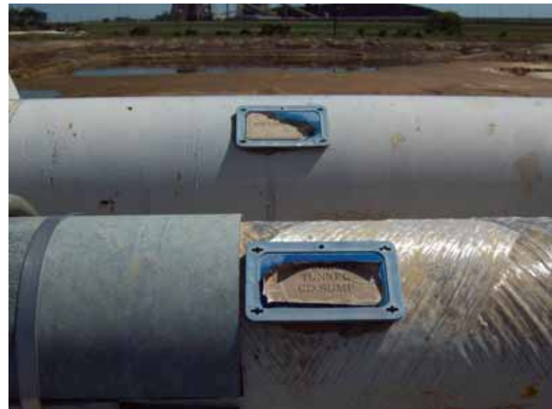
Photo 36: Labels for left two 6-inch-diameter inlets shown in Photo 34.
