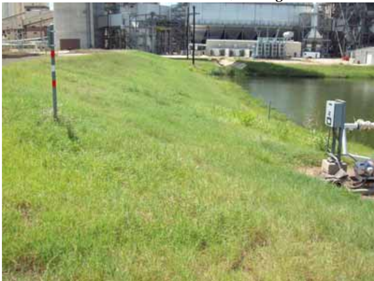
Photo 15: North embankment exterior slope, looking west. #1 Stormwater Runoff Pond at exterior toe.
