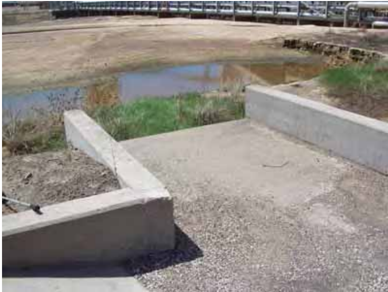
Photo 77: SP - Spillway between SRH Pond and South Bottom Ash Pond at west embankment exterior slope, looking west.
