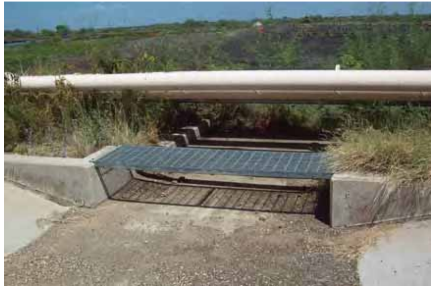
Photo 6: Spillway between SRH Pond and South Bottom Ash Pond at east embankment exterior slope, looking east.
