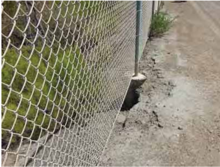
Photo 5: NP - North embankment exterior slope, looking northeast. Note erosion near fence post.
