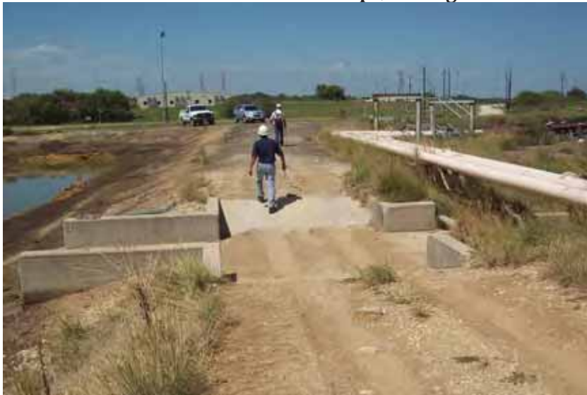
Photo 79: SP - Spillway between SRH Pond and South Bottom Ash Pond at west embankment crest, looking north.
