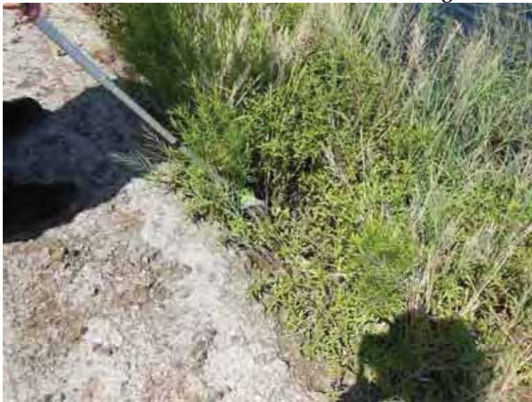
Photo 23: NP/SP - Erosion of ash material on common embankment north slope.
