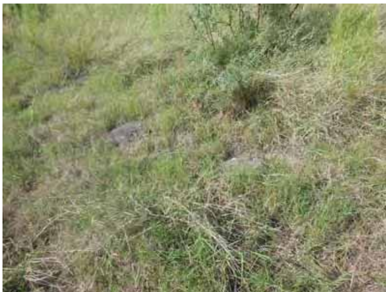
Photo 62: Loose soils on east embankment exterior slope.
