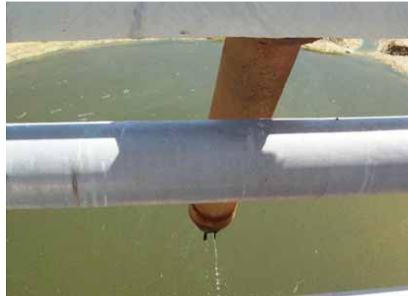
Photo 30: 6-inch-diameter metal SRH-south inlet pipe, looking south.
