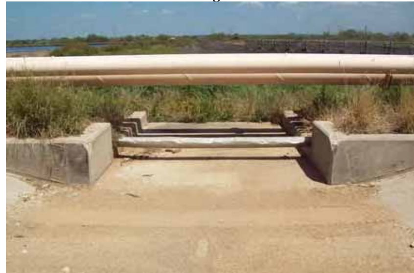
Photo 80: SP - Spillway between SRH Pond and South Bottom Ash Pond at west embankment interior slope, looking east.
