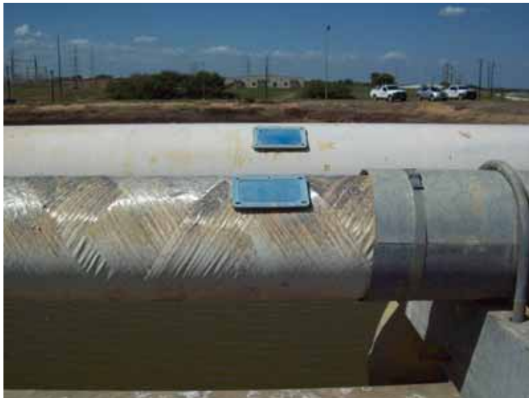
Photo 39: Labels for right two 6-inch-diameter inlets shown in Photo 38.
