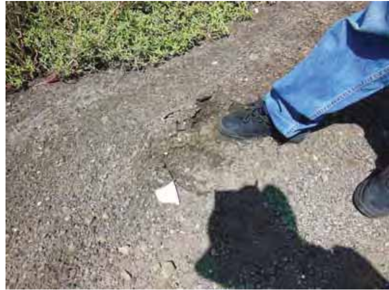
Photo 14: NP - Loose ash material at east embankment interior slope.
