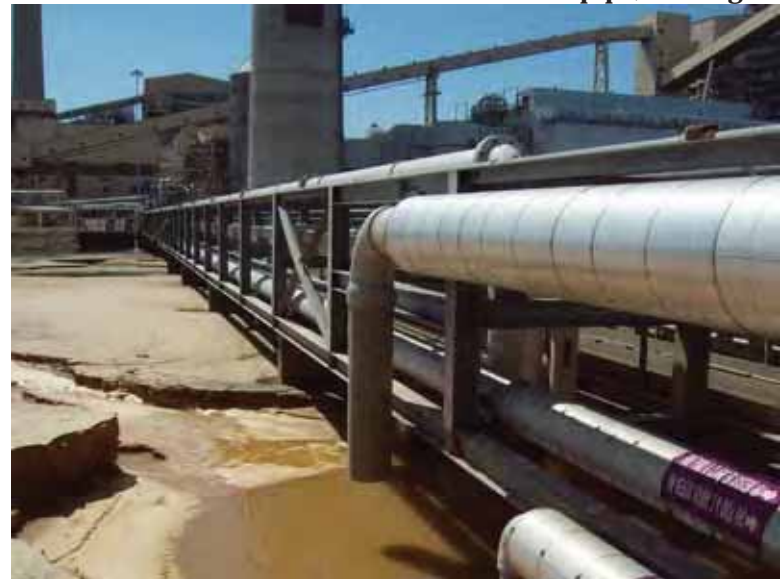
Photo 32: 8-inch-diameter SRH-south inlet pipe labeled “SRH Pond & Clarifier Syst 464”, looking west.
