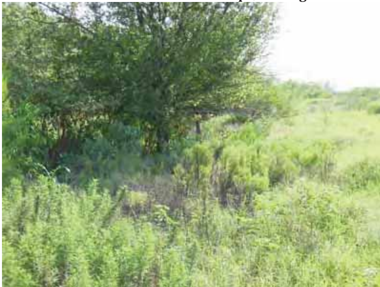
Photo 104: North embankment exterior slope, looking east. Note trees near exterior toe.
