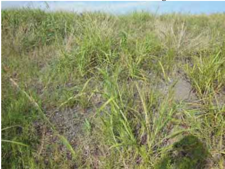
Photo 60: Loose soils on east embankment exterior slope.
