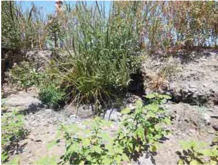
Photo 25: NP/SP - Vegetation and ash material on common embankment south slope.
