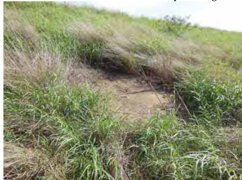
Photo 117: Exposed soil at south embankment exterior slope, looking north.
