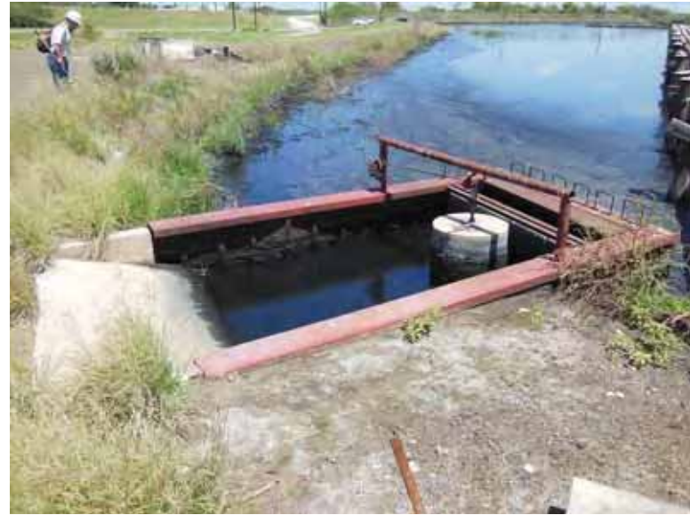
Photo 34: NP - 24-inch-diameter Plant return outlet, looking north.
