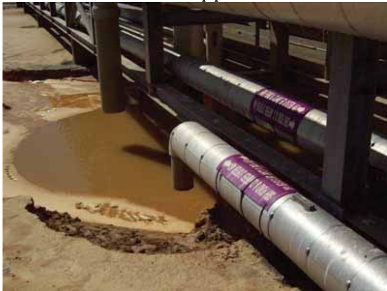
Photo 31: 6-inch-diameter SRH-south inlet pipe labeled “SRH Pond & Clarifier Syst 464”, looking west.
