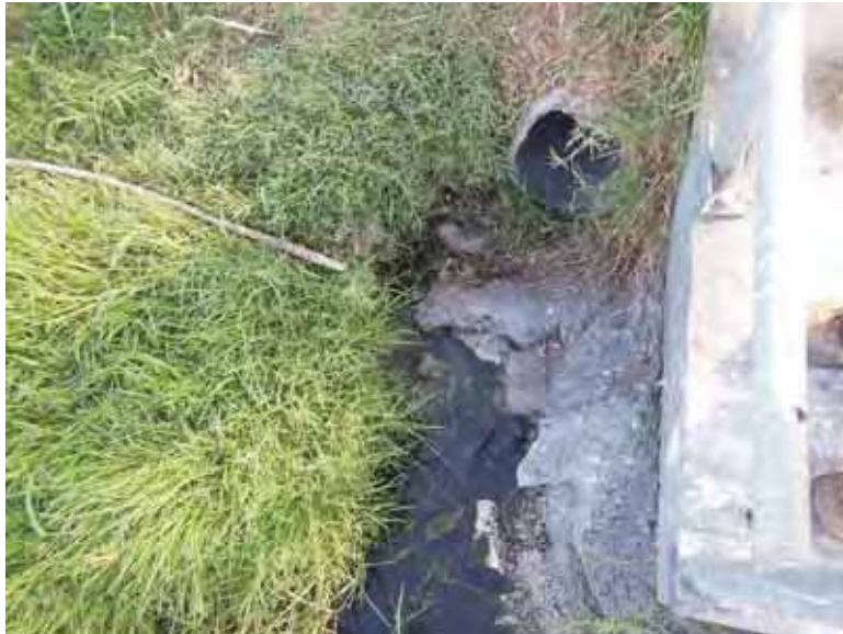
Photo 89: SP - 12-inch-diameter piping at outfall 103B.
