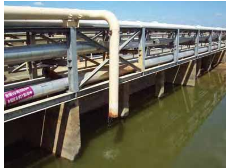
Photo 26: 8-inch-diameter metal SRH-south inlet pipe labeled "Plant Drain System III", looking northeast.
