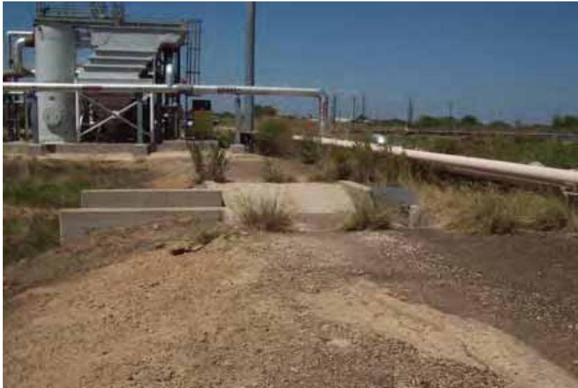
Photo 5: Spillway between SRH Pond and South Bottom Ash Pond at east embankment crest, looking north.
