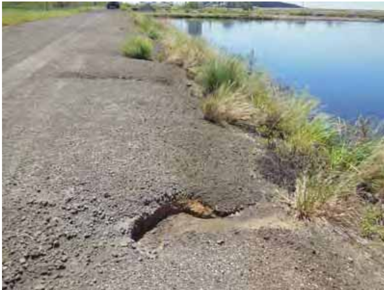
Photo 17: NP - East embankment interior slope, looking south. Note erosion rills in ash material.
