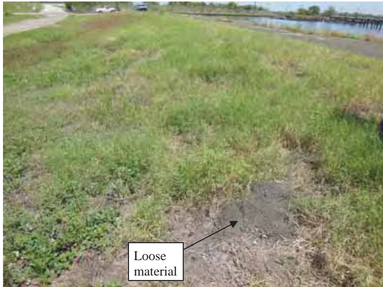
Photo 41: NP - West embankment exterior slope, looking north. Note area of loose soil/ash material.
