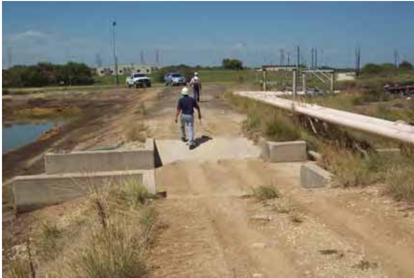
Photo 9: Spillway between SRH Pond and South Bottom Ash Pond at east embankment crest, looking north.
