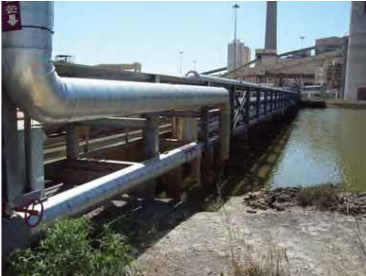
Photo 33: 6-inch and 8-inch-diameter SRH-north inlet pipe labeled “SRH Pond & Clarifier Syst 464”, looking west.
