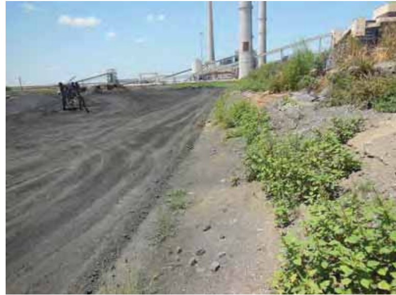
Photo 26: NP/SP - Erosion of ash material on common embankment south slope, looking west.
