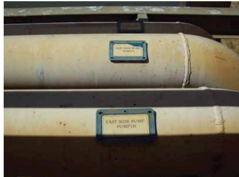
Photo 40: Labels for middle three 6-inch-diameter inlets shown in Photo 38.
