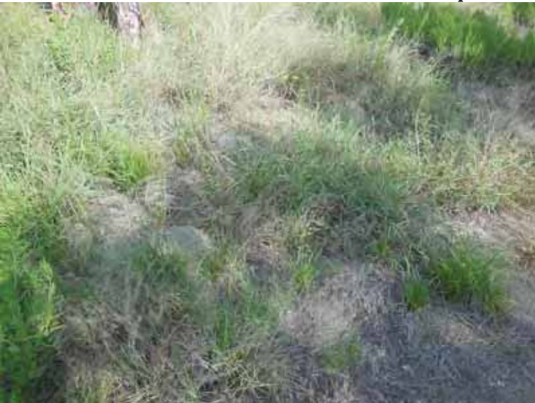
Photo 96: Loose soils near east embankment exterior toe.
