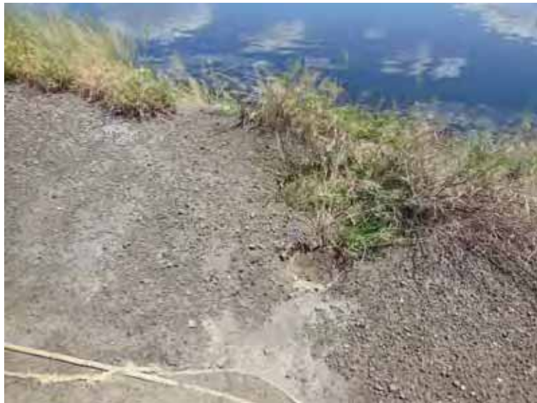
Photo 43: NP - Erosion of ash material at west embankment interior slope.
