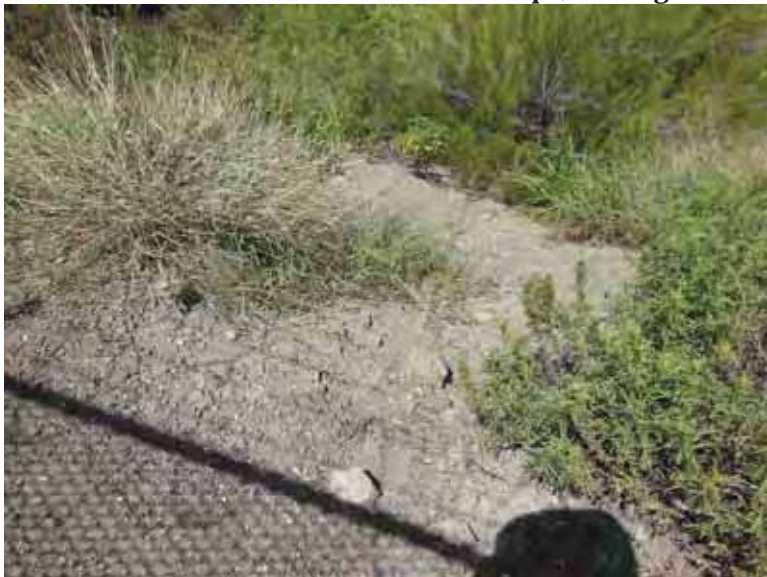
Photo 51: NP - Erosion on north embankment exterior slope, looking north.
