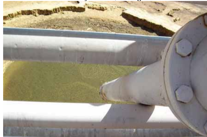
Photo 28: 6-inch-diameter metal SRH-south inlet pipe labeled "Waste Slurry Sump", looking south.
