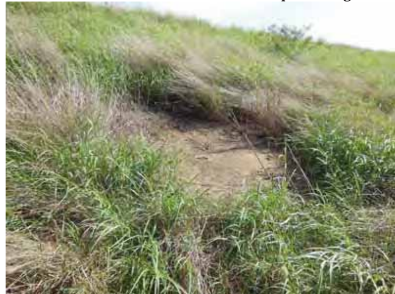
Photo 85: Exposed soil at south embankment exterior slope, looking north.
