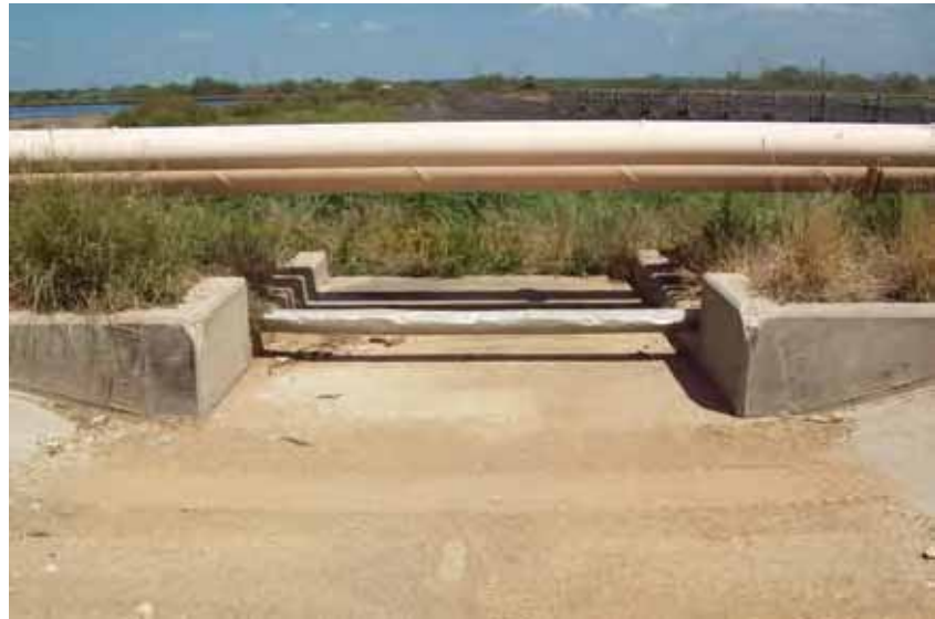
Photo 10: Spillway between SRH Pond and South Bottom Ash Pond at west embankment exterior slope, looking east.
