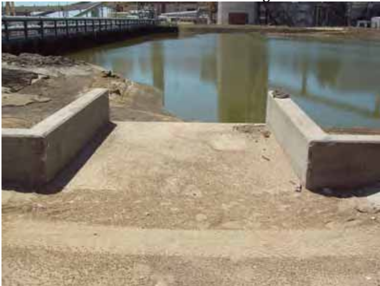
Photo 11: Spillway between SRH Pond and South Bottom Ash Pond at east embankment interior slope, looking west.
