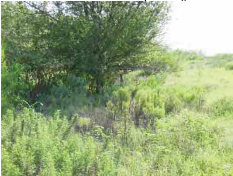
Photo 72: North embankment exterior slope, looking east. Note trees near exterior toe.
