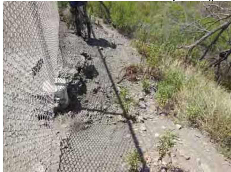
Photo 52: NP - Erosion at fence post on north embankment exterior slope.
