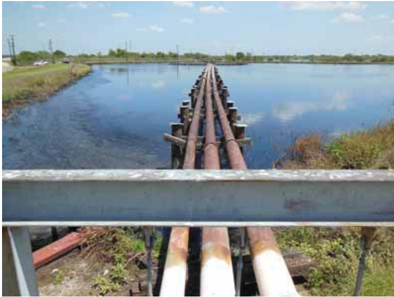
Photo 33: NP - Inlet pipes at southwest corner. Piping includes one 8-inch diameter and two 12-inch-diameter pipes.
