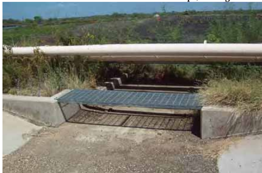
Photo 76: SP - Spillway between SRH Pond and South Bottom Ash Pond at west embankment interior slope, looking east.
