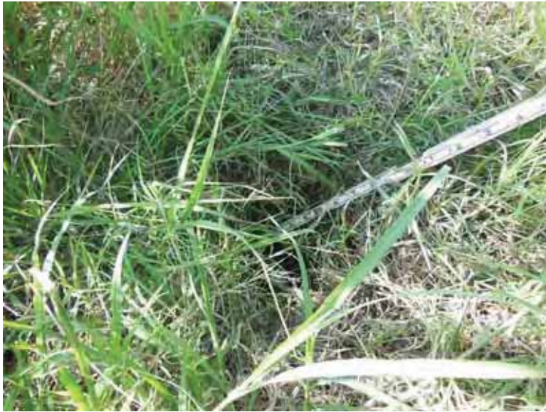
Photo 110: Approximately 18-inch-deep animal burrow at west embankment exterior slope.
