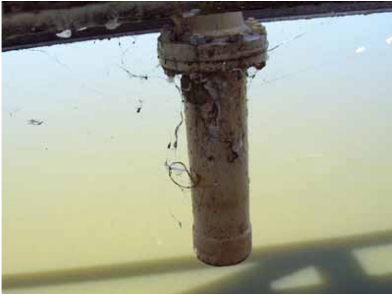
Photo 43: 6-inch-diameter metal SRH-north inlet pipe, looking north.
