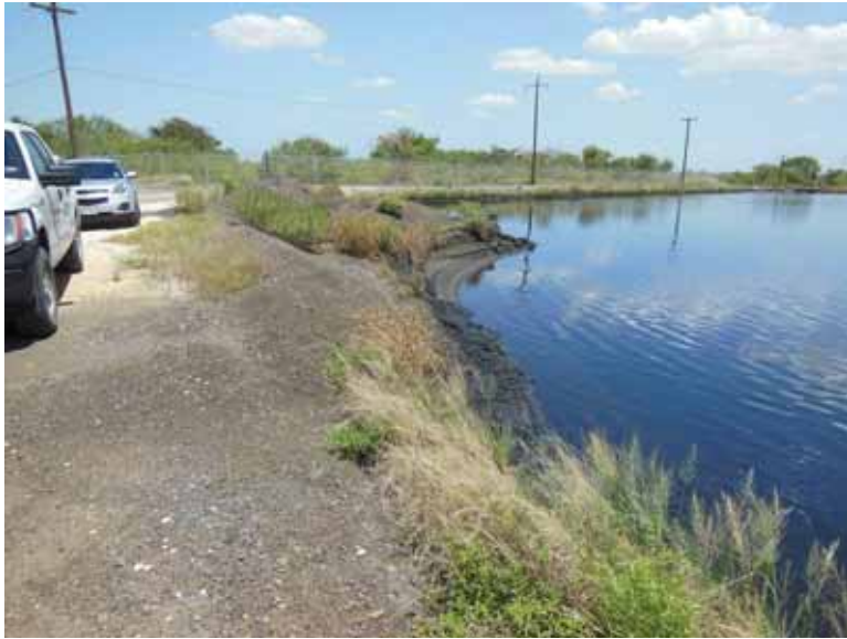
Photo 45: NP - West embankment interior slope, looking northeast. Note area of ash material on slope near northwest corner.
