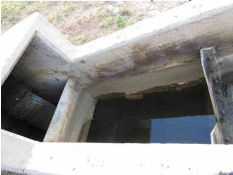
Photo 55: V-notch weir outfall for SRH Pond.
