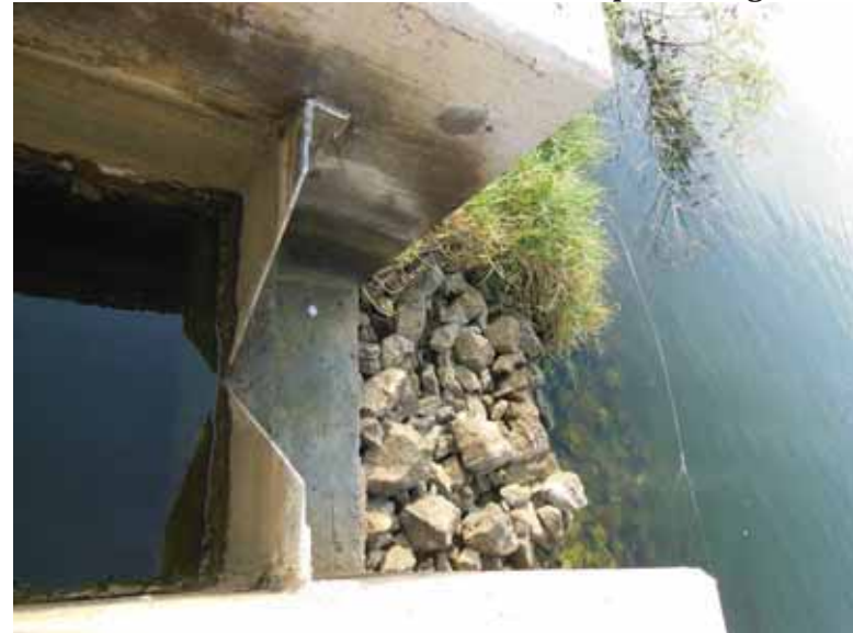
Photo 56: V-notch weir outfall for SRH Pond.
