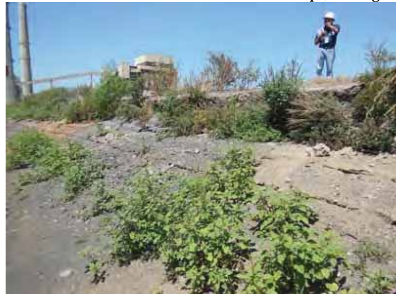
Photo 24: NP/SP - Erosion of ash material on common embankment south slope, looking northwest.
