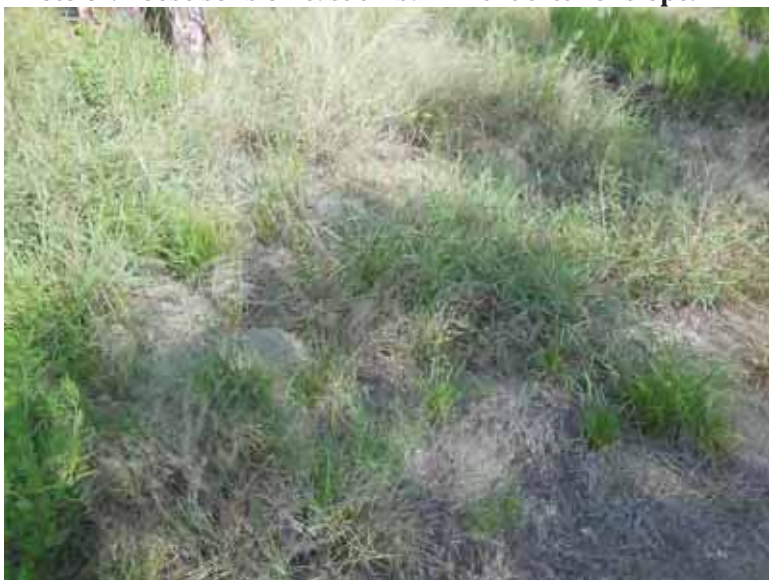
Photo 64: Loose soils near east embankment exterior toe.
