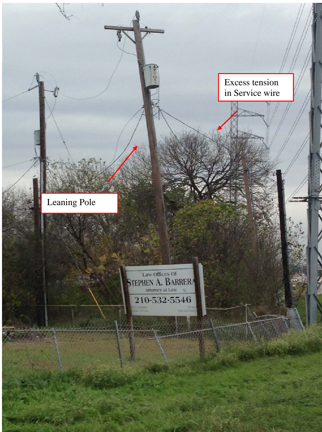
Figure 13 Pole with Excessive Lean
