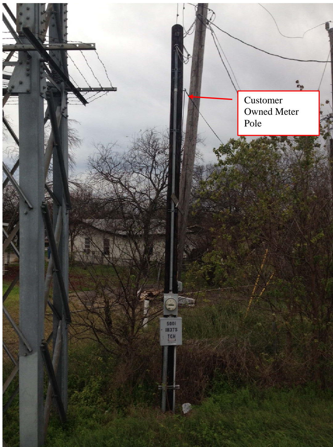
Figure 5 Customer Owned Pole
