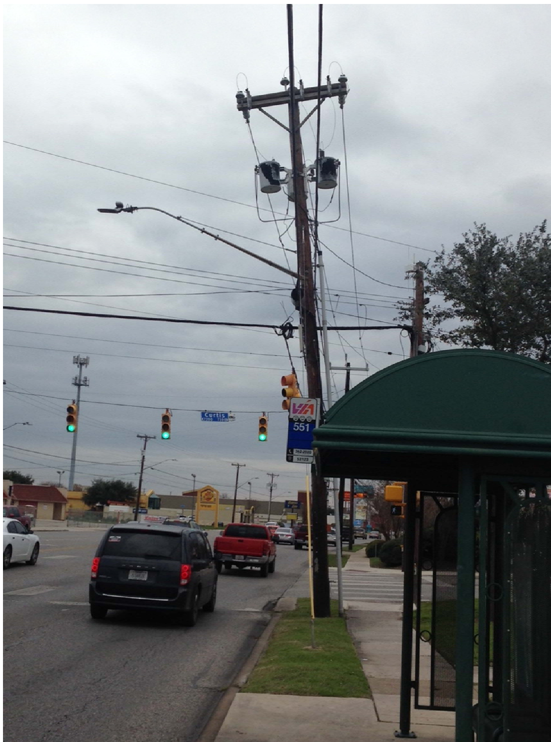
Figure 14 Three Transformer Pole with Excessive Lean
