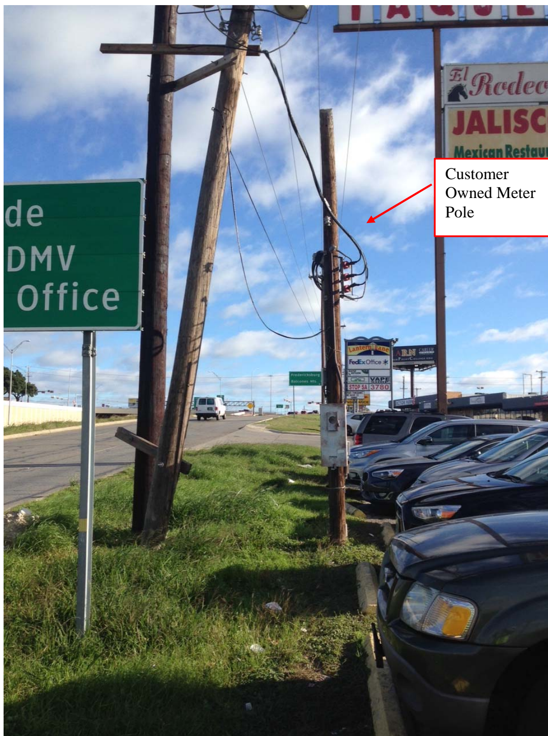
Figure 7 Customer Owned Pole for Commercial Service
