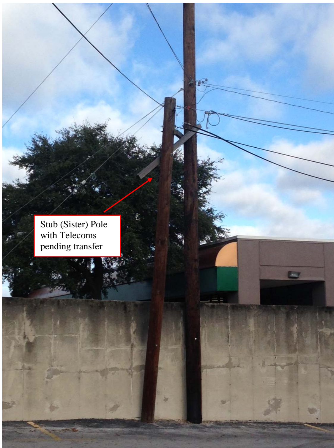
Figure 18 Stub (Sister) Pole with Telecom Cable Transfers Pending
