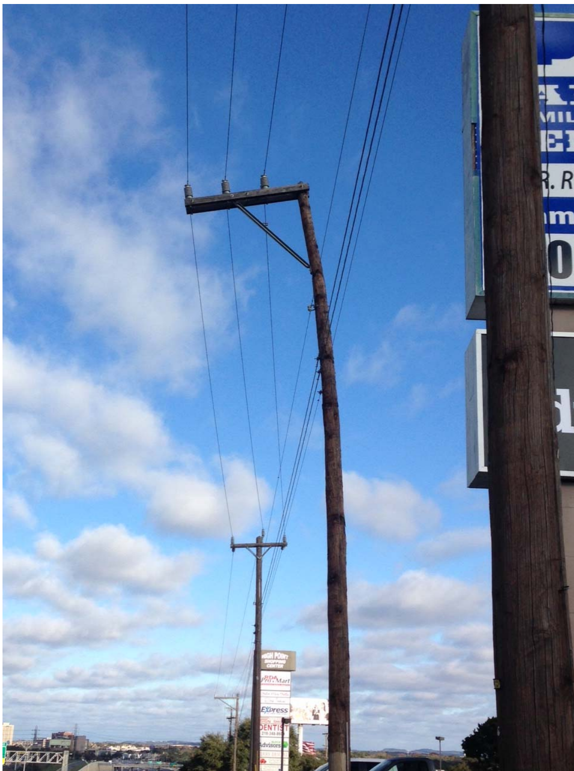
Figure 12 Pole with Excessive Bend at Neutral
