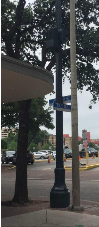
Downtown Wireless Streetlights
