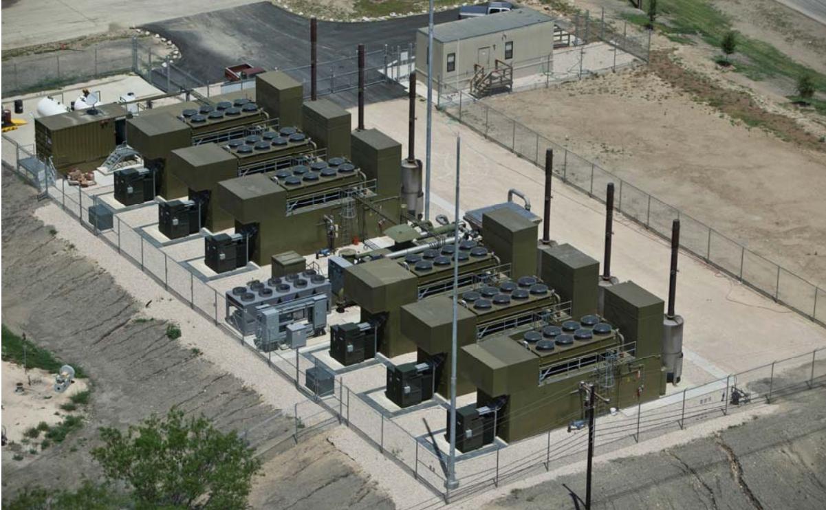
CPS Energy Landfill Gas Plant – Covell Gardens
