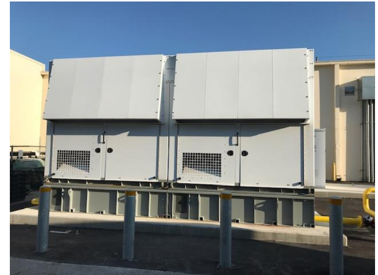
ERock natural gas generator at H-E-B
